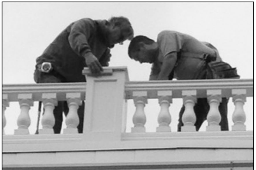
Mark Boschult (Boschult Engineering), left, and Josh DePatie (Moose Carpentry) tighten brackets that connect rail sections to the newel posts on the May Museum roof.
