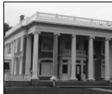
Work began last June on the roofline balustrade and now it looks like it did in 1901-02.
